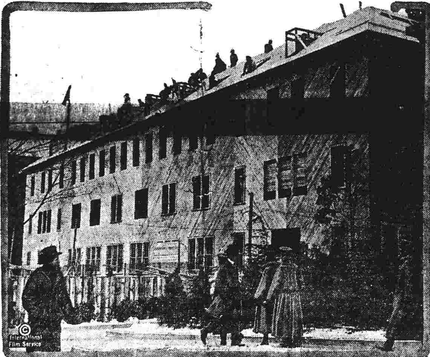
Three hundred workmen have been laboring at top speed to complete the new $100,000 building in Washington to serve as an annex to the navy department. The photograph shows the structure after twelve days' work.
